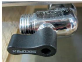
1. Control valve of steam generator
